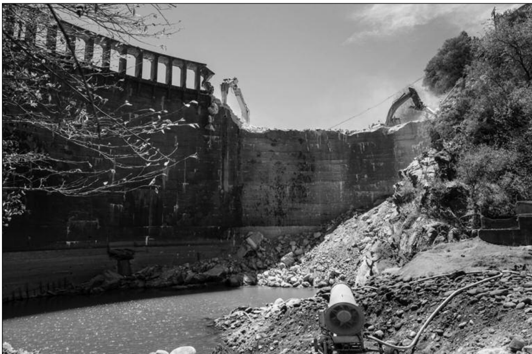
Removal of San Clemente Dam, summer 2015. Photo used with permission, California American Water.
