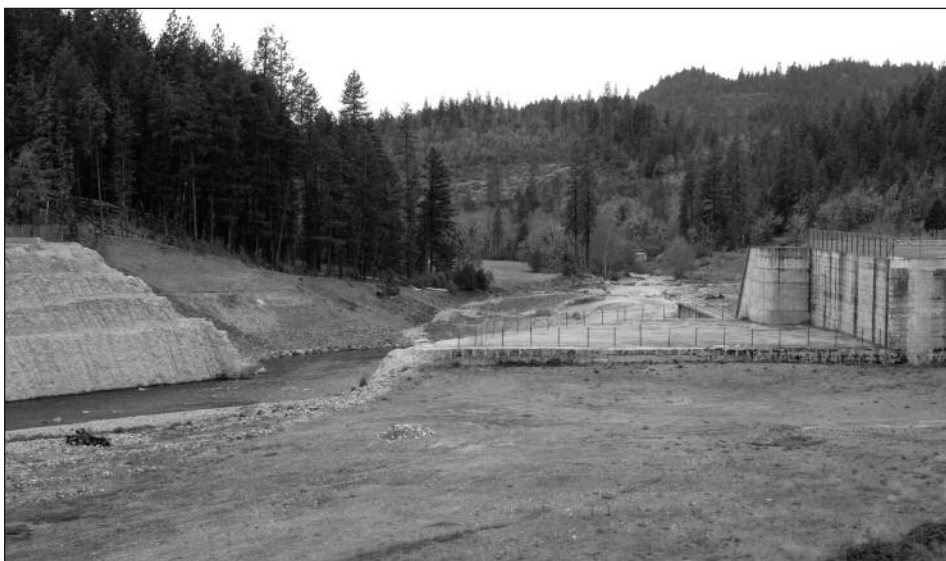
The partially constructed Elk Creek Dam blocked salmon and steelhead from important spawning habitat, while serving no useful purpose. It was notched in 2008, opening access to upstream habitat. Photo by Jim Yuskavitch
