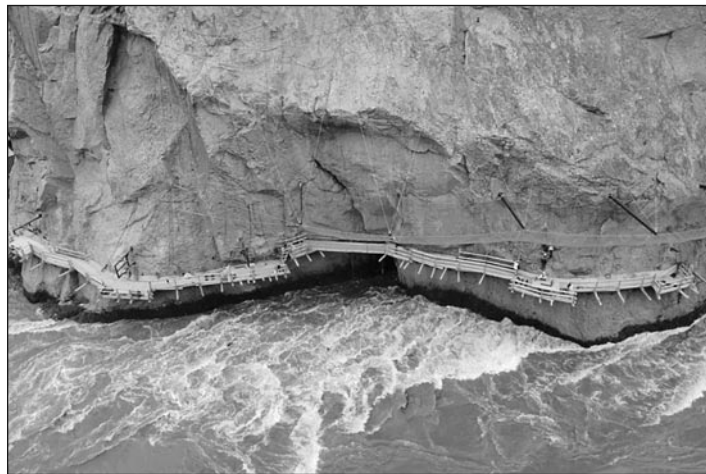
Passage portal construction at the Big Bar landslide site, Fraser River. Photo Courtesy Peter Kiewit Sons, ULC/Province of British Columbia. Attribution Non-Commercial 2.0 Generic License Converted to black and white
