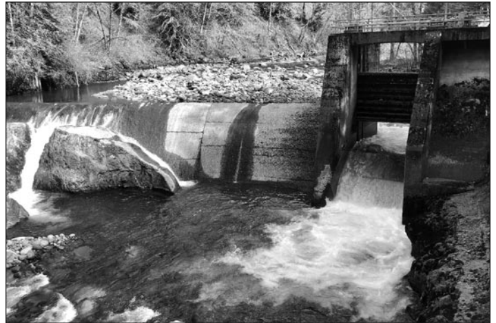
Removal of the Middle Fork Nooksack Dam has opened 16 miles of previously inaccessible habitat to salmon and steelhead. Photo by April McEwen/American Rivers
